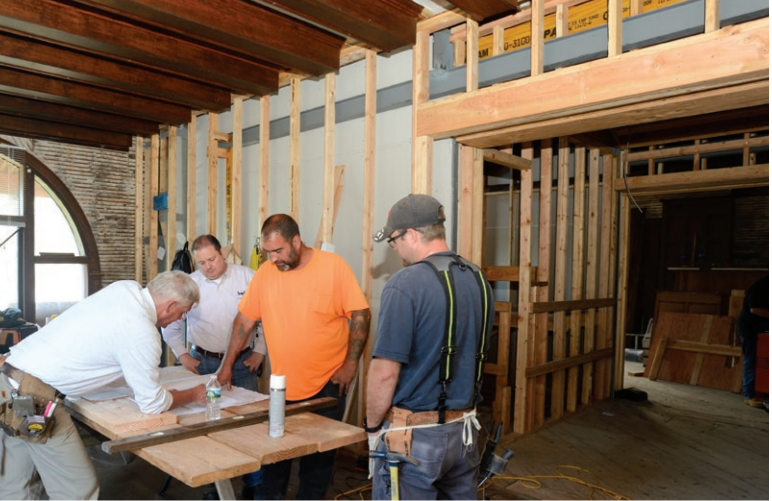
Bauer Hall, currently being renovated, will house the Innovation Center to provide resources and expertise to student-entrepreneurs like David Alvarez.
